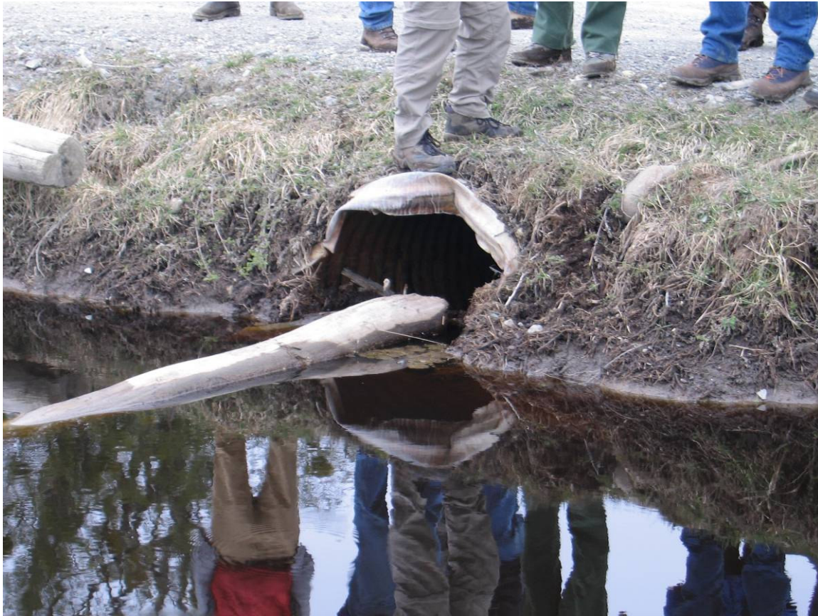
Fig. 5 Beaver attempts to block a road culvert, Tolhuin, Tierra del Fuego.
